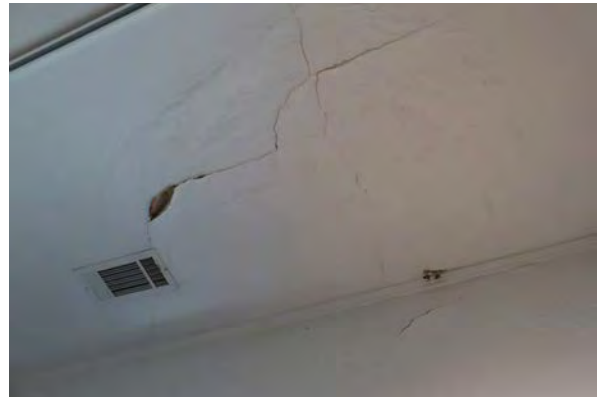
Water damaged ceiling and wall in southeast room.
