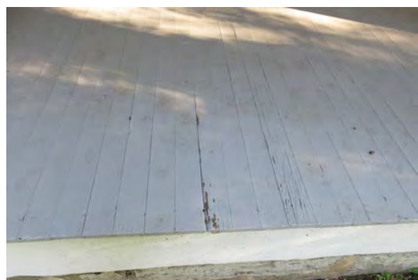
Damage and deterioration at tongue and groove floor at the first floor.
