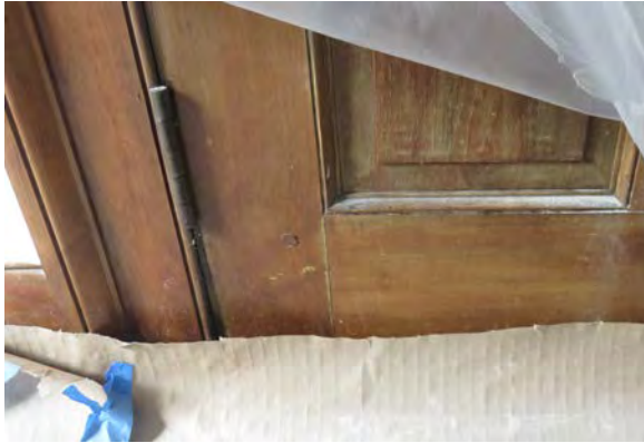
Water damaged finish at door to the north elevation in the first floor west room.
