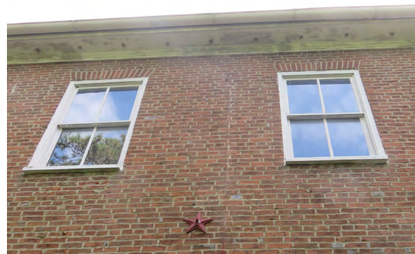
Second floor windows at the west elevation, showing signs of paint deterioration at bottom rail of upper sash.
