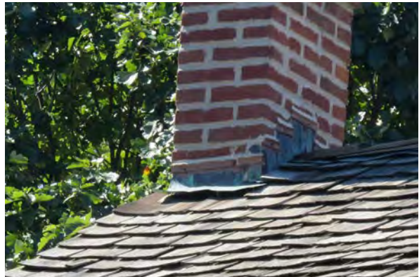
Lifting flashing at south chimney. Note the deteriorated sealant.
