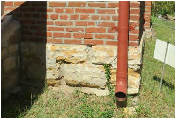
Open joints and previous repointing efforts at the ashlar foundation.
