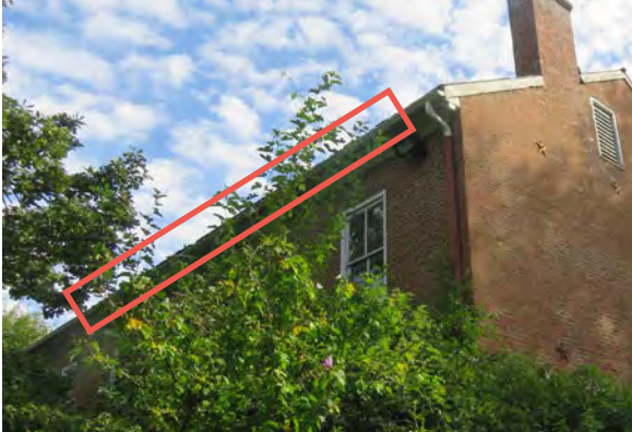
Area of damaged gutter outlined in red. Note you one can see the edges of the shingles due to the bent gutter.
