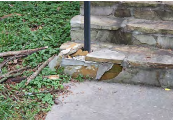
Damaged corner of northwest stair. Note that this area has been repaired, but that repair has failed.
