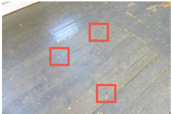
Repaired holes in the floor in the second floor east room, outlined in red.
