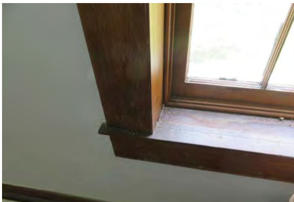
Water damaged finish at window sill from previous water infiltration issue.
