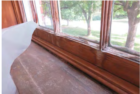
Water damage at new sash, deteriorating finish at window sill.
