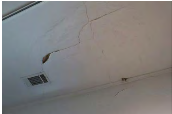
East Building. Water damaged ceiling and wall in southeast room at the second floor.
