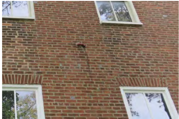
Pipe at the north end of the west elevation leaking an unknown substance down the brick.
