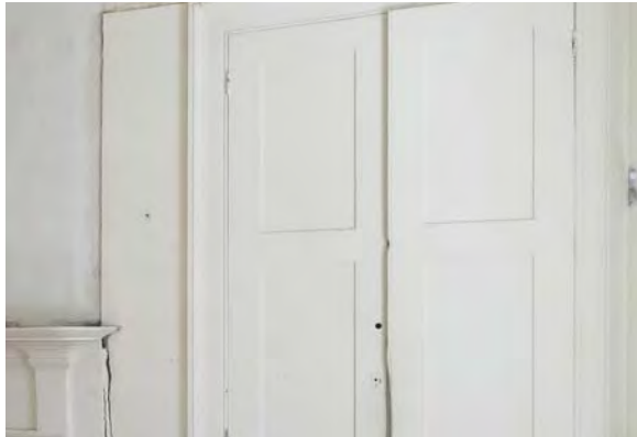
Missing and over-painted hardware on built-ins.
