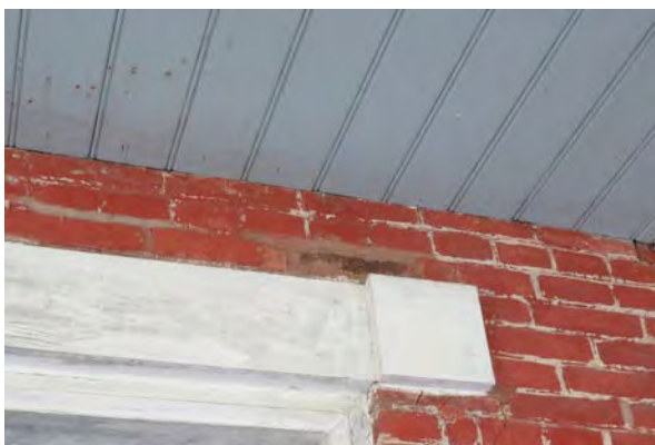
Previous repair that does not match the adjacent masonry.
