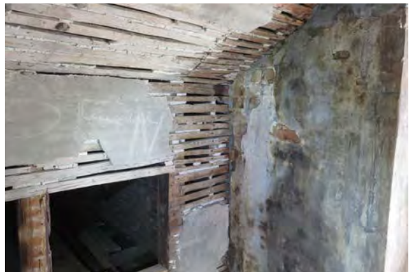
Plaster and lath in the attic at the south end. Note the graffiti scratched into the plaster on the left.
