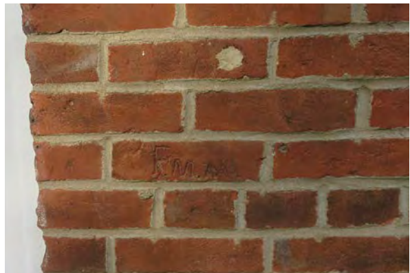
Scratched initials in the brick face. Note the mortar patch a few courses above.
