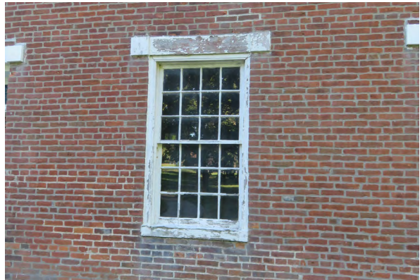
Window with heavy paint and glazing putty deterioration. This window does not appear to have been included in the 2016 scope.
