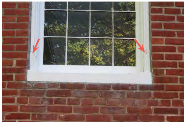
Repaired window where seams from dutchman repairs are visible through the paint. Note the unpainted grey sealant at the edges of the window frame.
