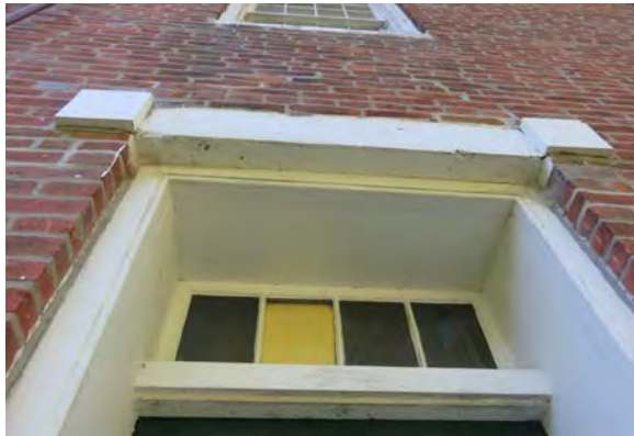
Transom with opaque replacement glass at the northwest door.
