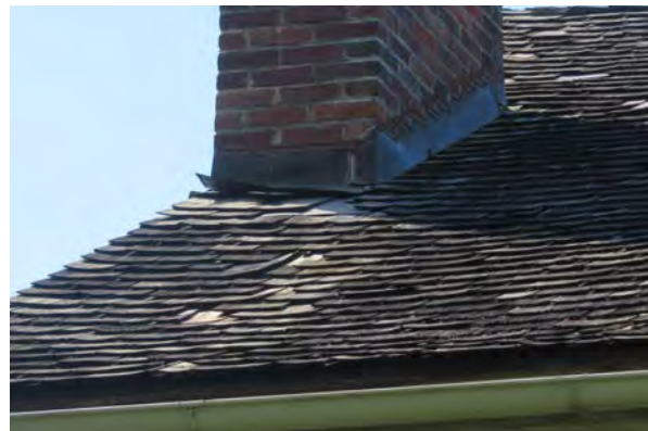
Lifting flashing and deteriorated sealant at southeast chimney.
