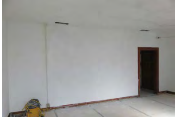
New wall at second floor west room. Note that this floor slopes to the center of the room.
