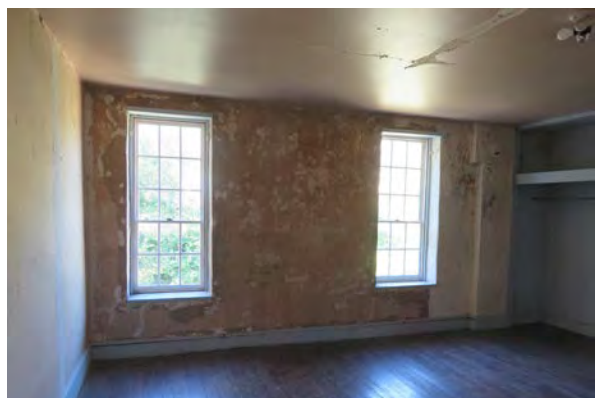
Plaster wall at second floor room in the rear addition. Note the ceiling damage and unfinished drywall on the left.
