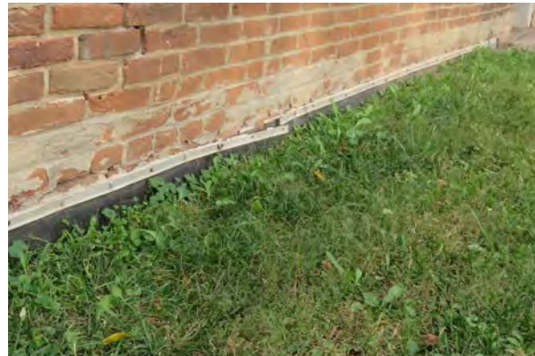
Location of the waterproofing membrane pulling away from the masonry.
