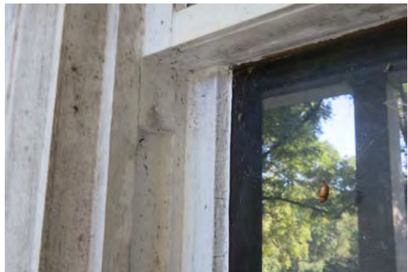
Window at the porch that is painted closed.
