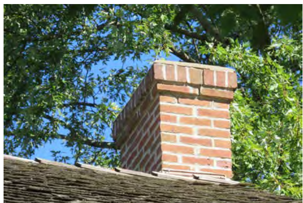
Cracks at mortar cap and open joint at chimney.
