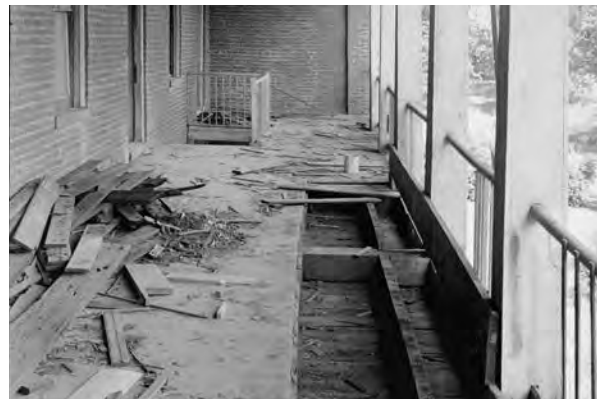
1940s HABS photo showing missing porch floor at the second floor.
