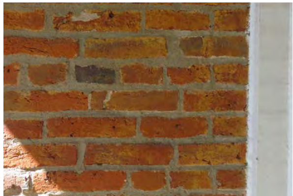
Brick with traces of yellow coating.
