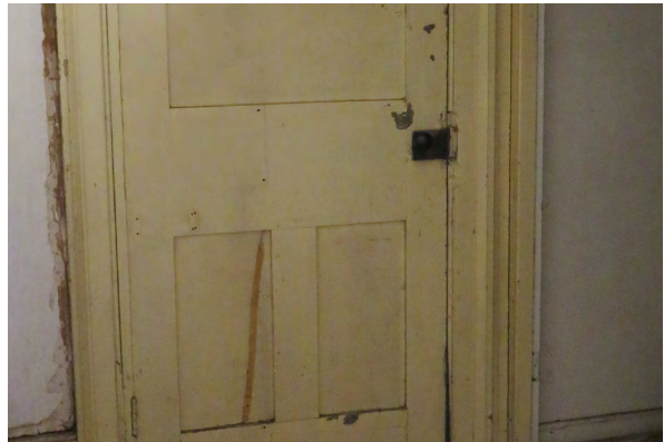
Old box lock on the porch door. Note the repaired wood check in the lower left panel.
