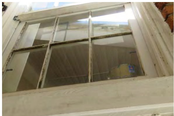
Deteriorated paint and glazing material at a window on the south elevation.
