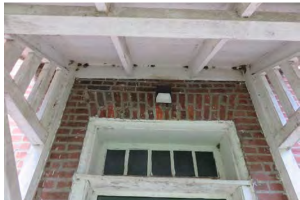
Deteriorated paint and insect nests below awning. Note the overpaint and deteriorated paint at the door surround.
