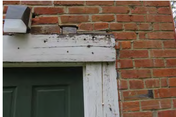
Wood and paint deterioration at kitchen door.
