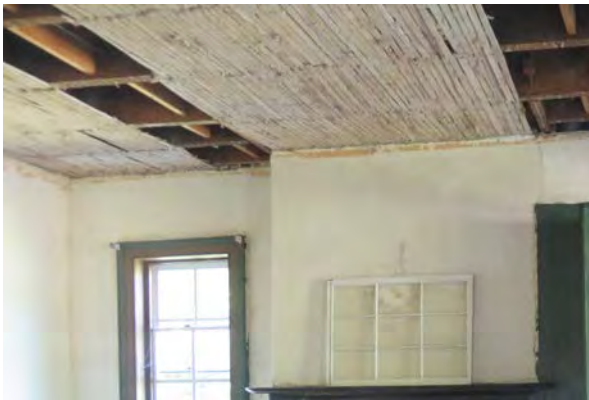
West Building. Missing ceiling in the first floor west room. Note the ghosting from a crown molding.
