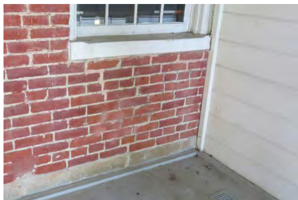
Open joints below window at the porch.
