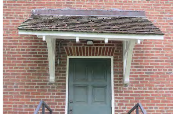
Sagging awning at the northwest entrance. Note the failed sealant at the flashing above the awning.
