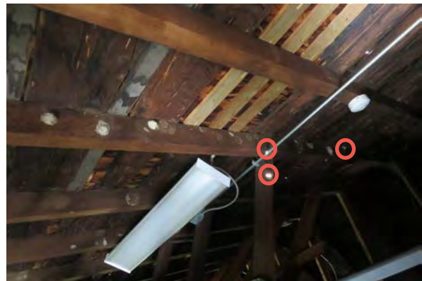
Roof from attic. Note the new sheathing boards. Spots of daylight coming through the roof are circled in red.
