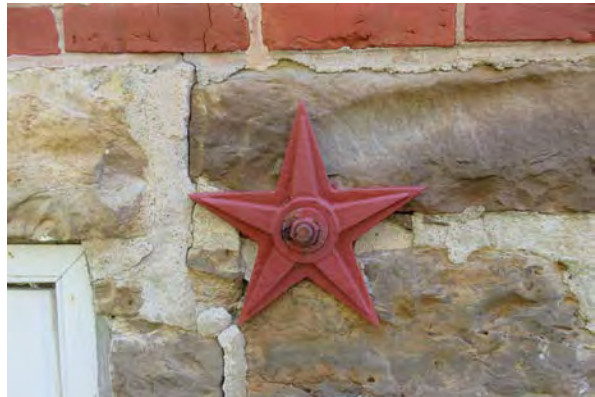
Paint deterioration and rust at building tie.
