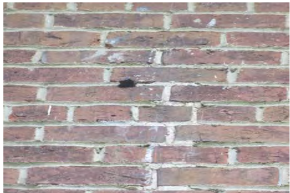
Old anchor and staining from old downspout location.
