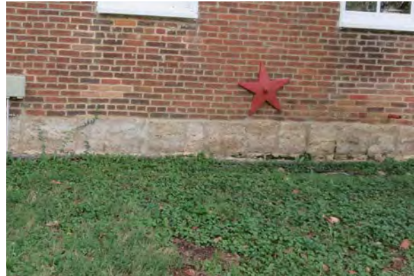
Open joints and plants growing in the gaps of the stone foundation.
