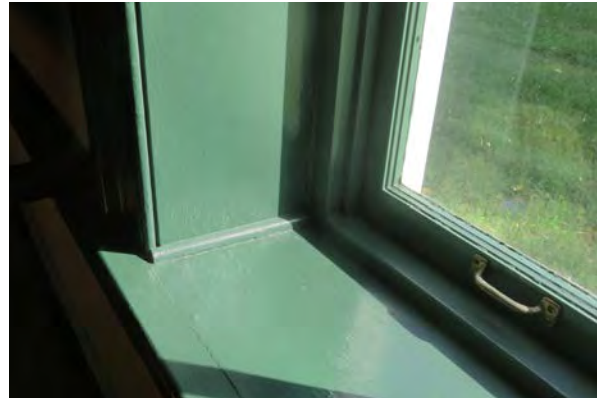
Windows on the first floor did not open and appear to be painted shut. It is unclear if this was intentional or due to high temps and humidity during the site visit.
