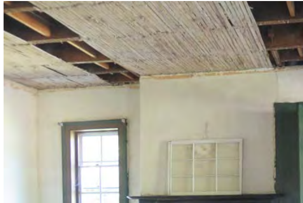
Missing ceiling in the west room. Note the ghosting from a crown molding.
