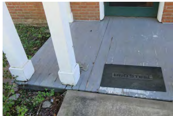
Paint and wood deterioration at north porch. Note the open seams in the column bases. These conditions are typical of both porches.
