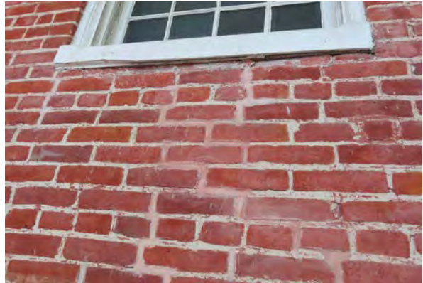
Area of repointing that does not match the rest of the masonry. Note the traces of red coating on the masonry on the right side.
