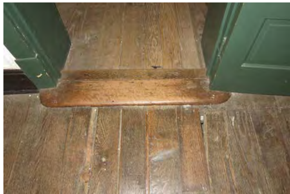
Large threshold at south door to second floor central room, due to floor slope. Note the broken board to the right.
