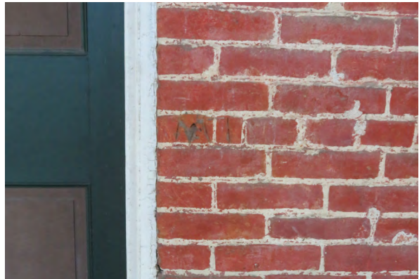
Scratchiti on brick.
