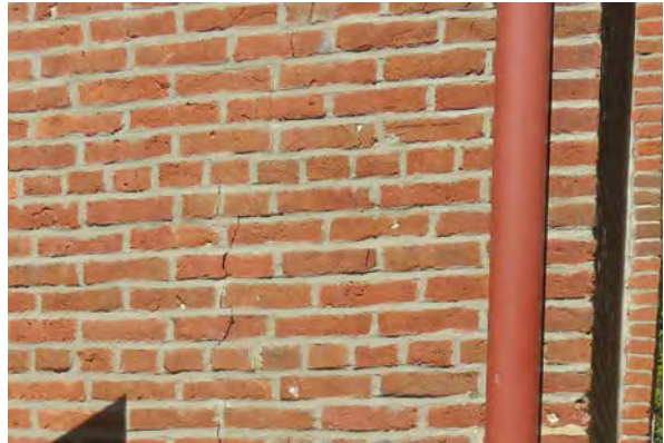
Masonry crack at southeast corner.
