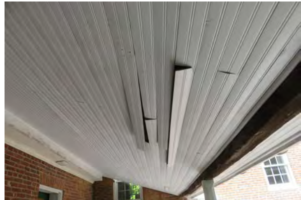
Falling cladding at the second floor of the east porch.
