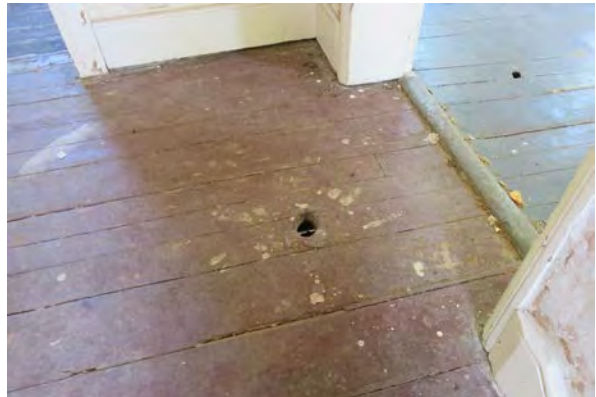
Holes in the floor of the second floor landing and second floor east room.
