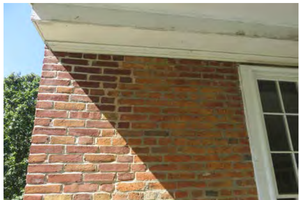
Repointing at an area of brick replacement. Note the different colors of mortar and the yellow coating on the bricks to the right.
