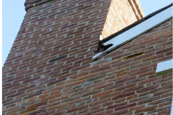
Hole in fascia panel on west elevation.
