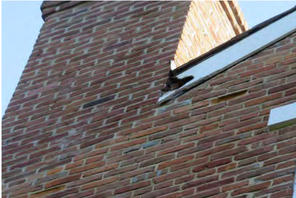
North Building. Hole in fascia panel on west elevation.
