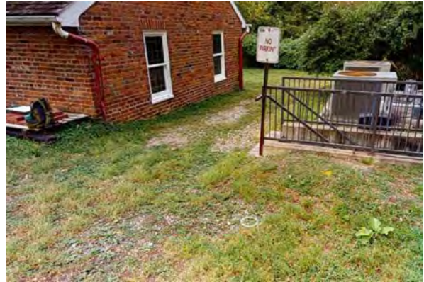
Area with thin gravel cover. Piping from the downspout in this corner can be seen through gravel in some areas.
