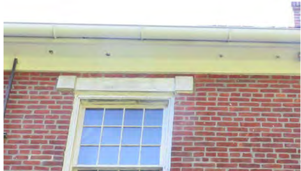
Painted over vents at the soffit underside.
