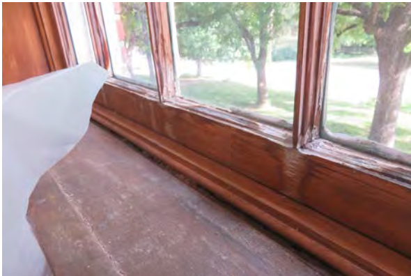
North Building. Water damage at new sash, deteriorating finish at window sill.
