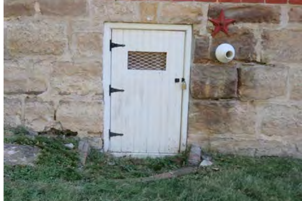
Open joint around cellar door.
