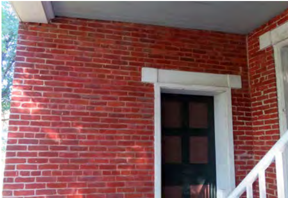
Masonry. Note the red coating on the brick, which has worn off most of the mortar joints.
