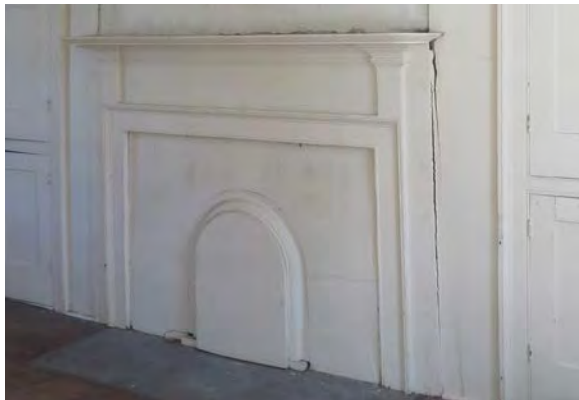
First floor east room fireplace and mantel. Note the separation at the right side.
