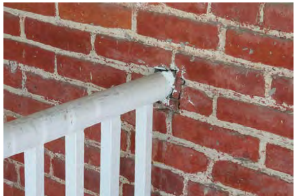
Rail termination at the masonry. Note the wood blocking added to stabilize the railing.
