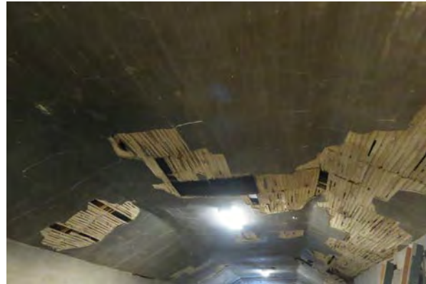
Plaster ceiling at the attic. Note staining and large areas of missing plaster and missing lath.
