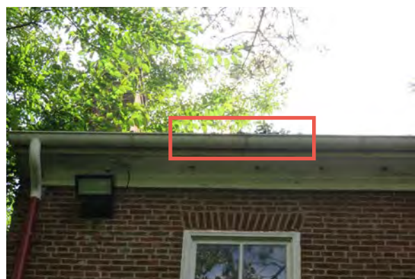
Pine needle and plant buildup in gutter visible from ground level, outlined in red.
