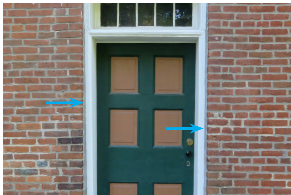
Unpainted grey sealant added at the door surround.
