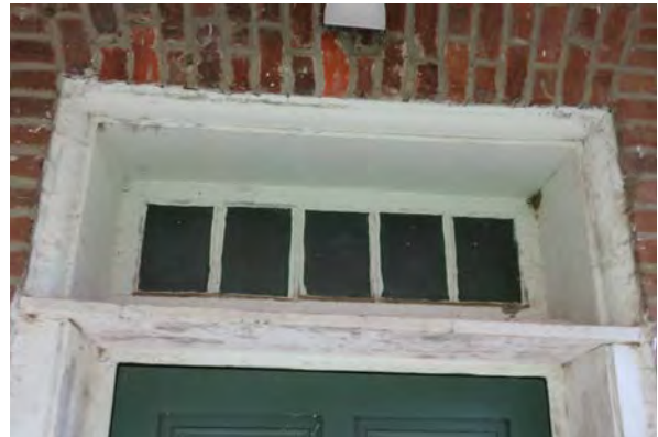
Deteriorated sealant at door surround.
