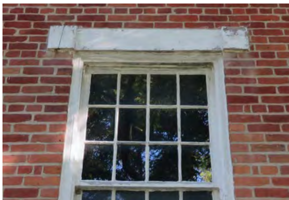
Paint and wood deterioration at flat lintel and raised wood block detail.
