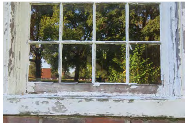
Paint and glazing putty deterioration at a north elevation window.
