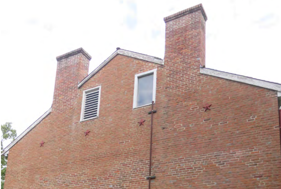
Deteriorated paint at south fascia.
