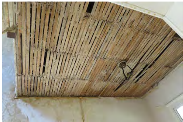
Exposed lath in foyer.
