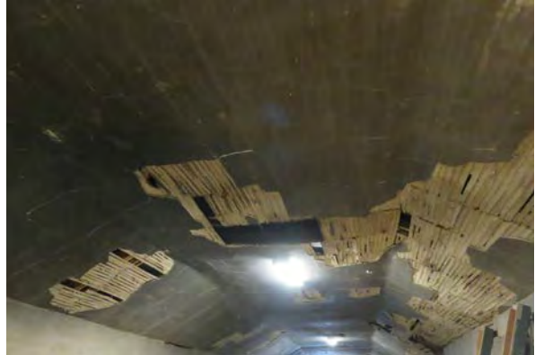
East Building. Plaster ceiling at the attic. Note staining and large areas of missing plaster and missing lath.
