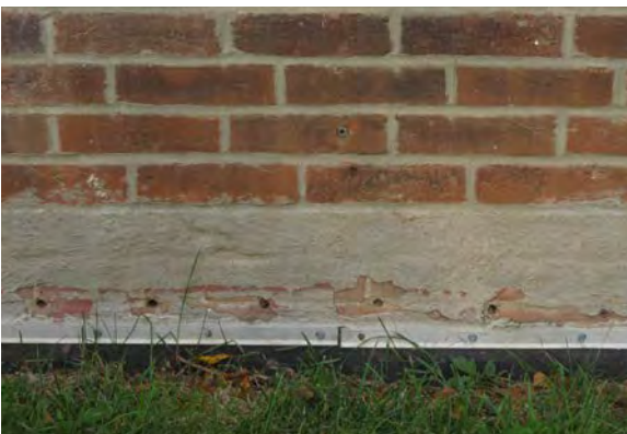
Cement parging and abandoned anchor holes above waterproofing membrane at the east elevation.
