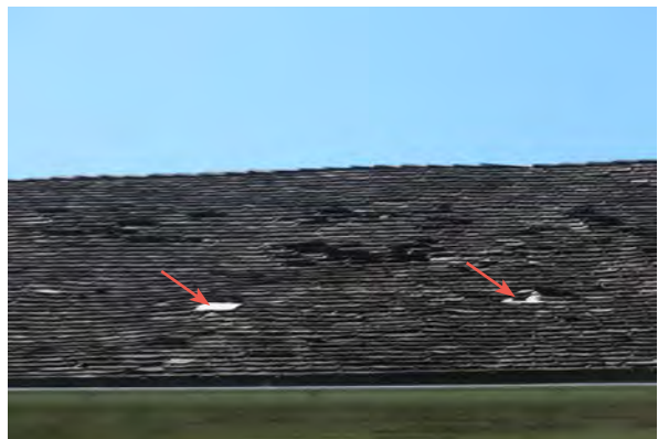
Lifting and curling shingles. Note the plastic sheets used instead of shingles, indicated with red arrows.
