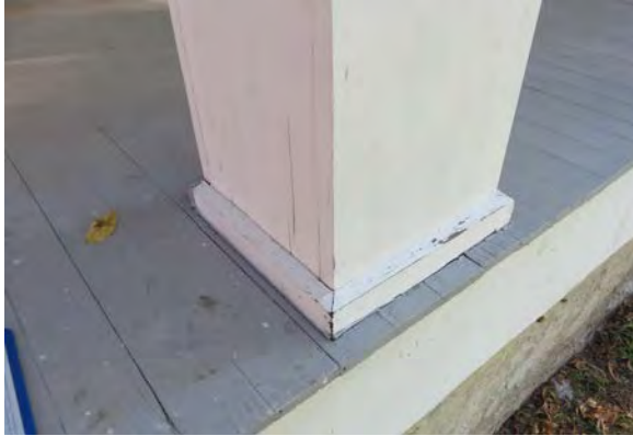
Paint deterioration, checking, and open seams in wood trim at column bases.
