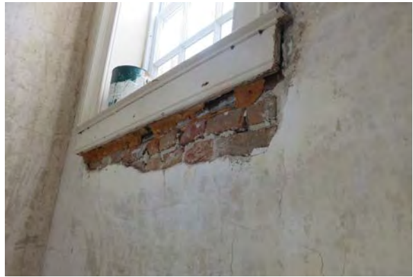
Plaster damage and exposed masonry below stairwell window.
