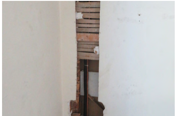
Opening in rear addition south room showing lath behind wallboard.
