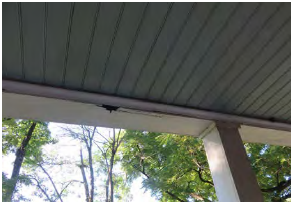
Wood deterioration at porch soffit.
